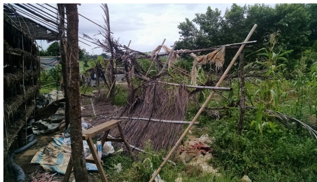
Figure 5. A mushroom house roof that was damaged in a storm.
