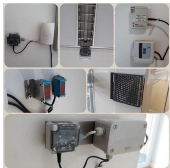
Fig. 2. Installed room sensors.
